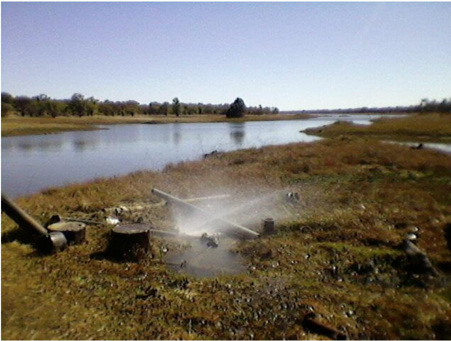
Picture 1: Old leaking irrigation mainlines at Doreen's Pride estate
